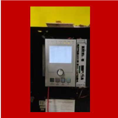
Edwards Fire Alarm Systems
