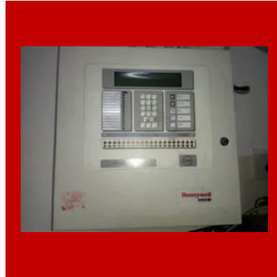
Morley Fire Alarm Systems
