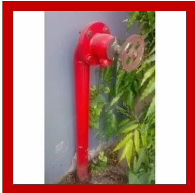
Fire Hydrant Valve
