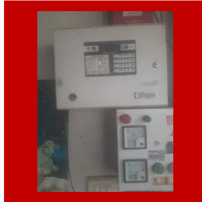
Fire Alarm System Installation Service
