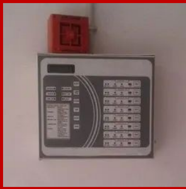
Agni Fire Alarm Panel
