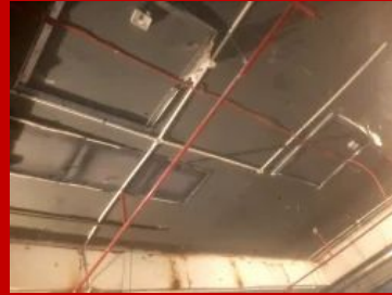
Fire Sprinklers System
