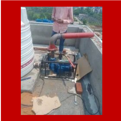
Fire Hydrant Pumps
