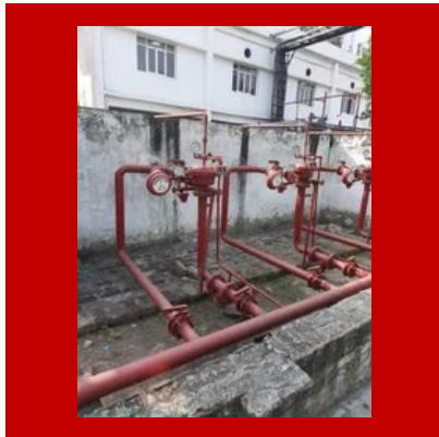
Fire Suppression Systems
