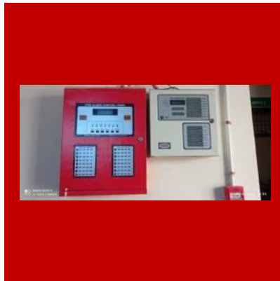
Fire Control Panel
