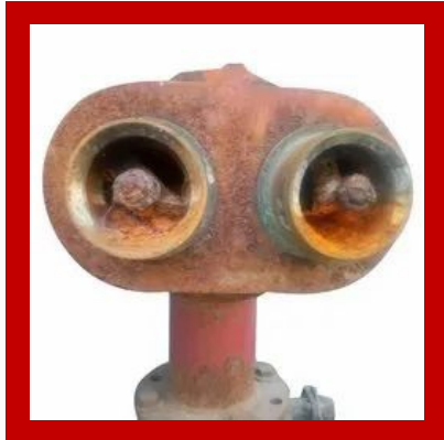
Fire Hydrant Two Way Inlet Breeching Valve
