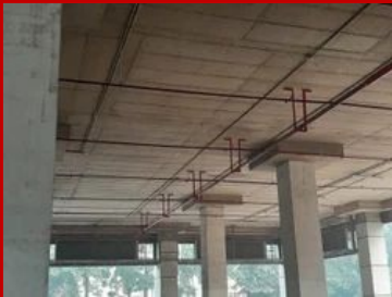
Fire Sprinkler System
