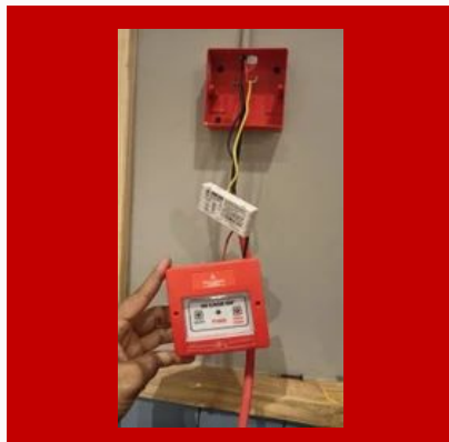
PVC Double Zone Fire Alarm
